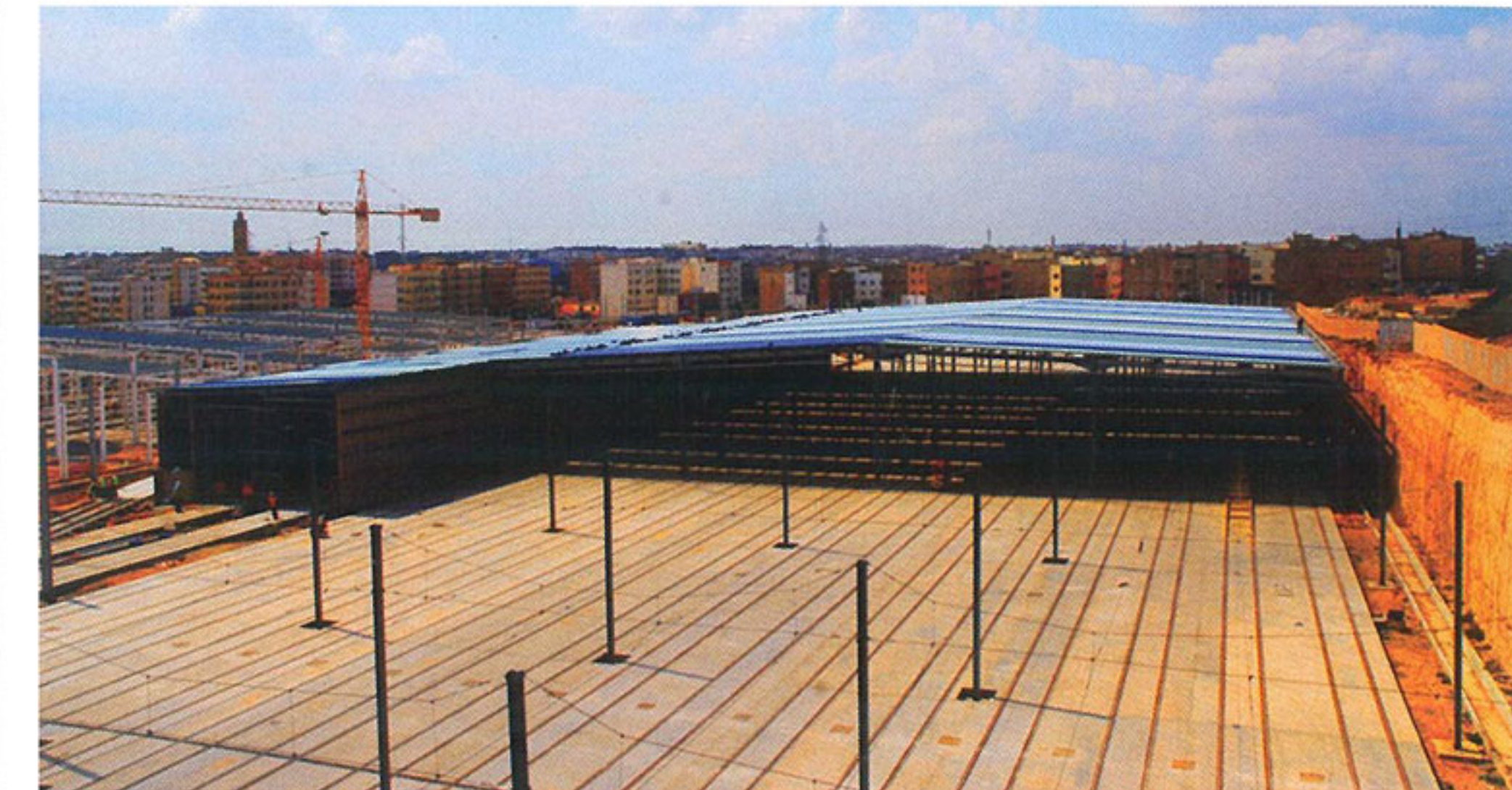
Above: The depot near Sidi Moumen includes a control centre and administrative offices.
